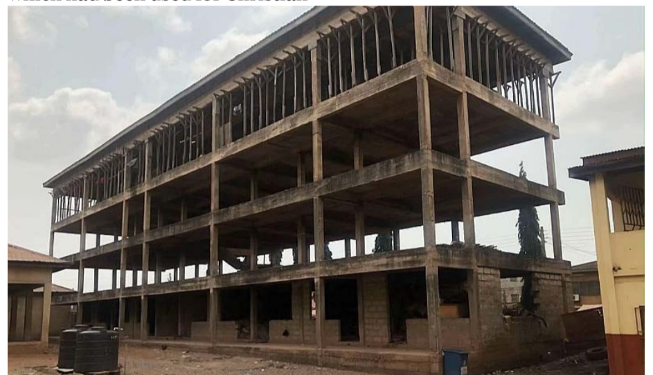
The state of the building before it collapsed
