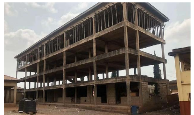
The state of the building before it collapsed
